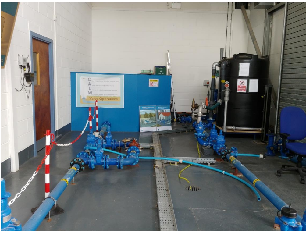
Figure 8: Balmore WTW Training Centre Pressure Transient Training Rig (photo by Isle Utilities)
